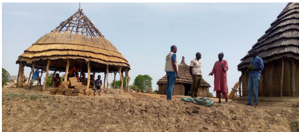
Household in Abyei Chock raising a plinth to 1.5m to protect from floodwater.
